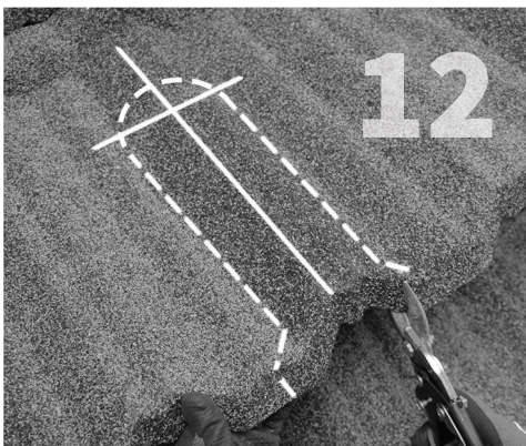
Cut an opening around the cone flashing and down to the bottom of the 1/2 length panel.
