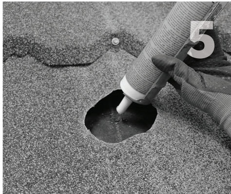
Add sealant compatible with contacted materials and environmental conditions to the pilot holes.
